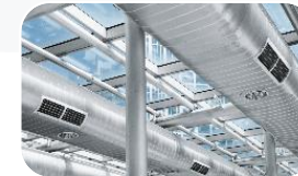
Heating Ventilation, & Air Conditioning (HVAC)
